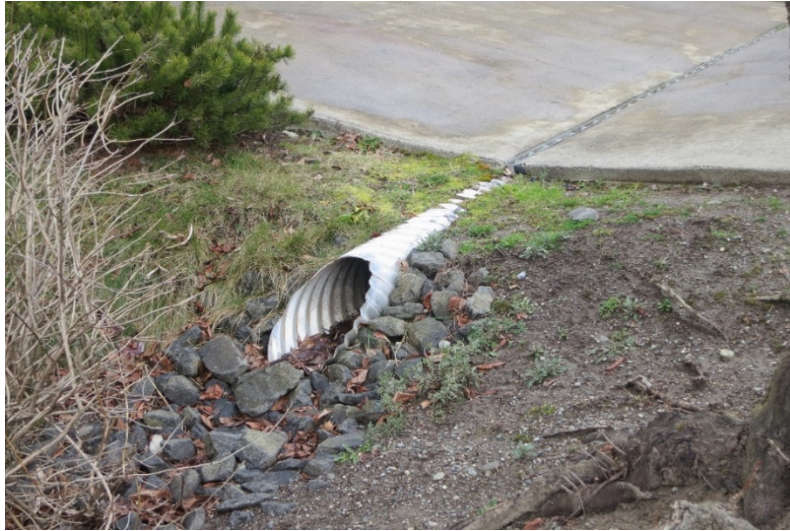
Water from the sloped driveway empties to a bioretention area
