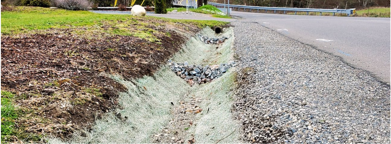
Figure 7. Drainage ditch with erosion control matting and rock check dams to slow water conveyance. Credit C. Thompson
