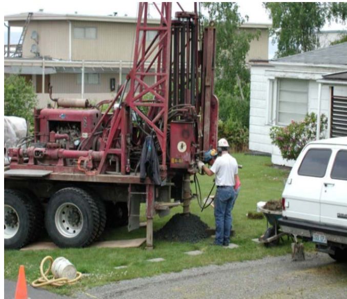
A boring machine digging deep on a site for site infiltration exploration
