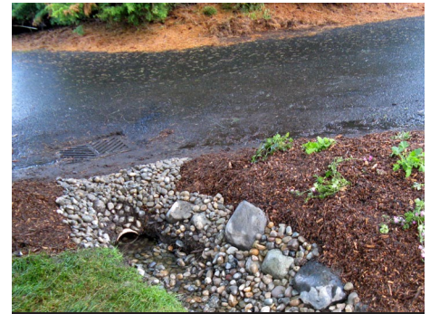
Applying clean drain rock to inflows and overflows prevents erosion and siltation of the rain garden.
