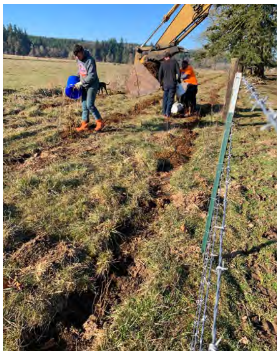
▲ Mulch is especially important in a hedgerow's early years. During monitoring visits, ensure that bare ground is covered, especially before fall rains that can cause erosion and dispersion of weed seeds in spring. Existing farm equipment can be useful to move mulch close to where it's needed, saving labor time. (Photo: Kevin Jensen)
