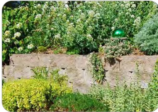
Retaining walls can be an effective solution to create level areas for planting while protecting steep soil excavations from erosion.
