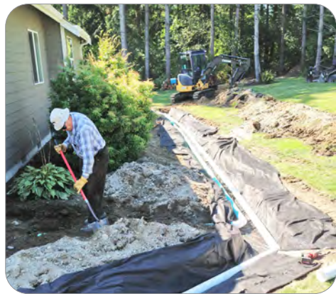
Size your infiltration system using the square footage of the area you plan to infiltrate and your soil texture.
